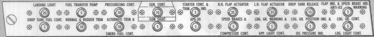
LEFT-HAND FORWARD CONSOLE CIRCUIT-BREAKER PANEL
