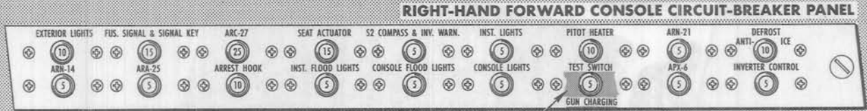
RIGHT-HAND FORWARD CONSOLE CIRCUIT-BREAKER PANEL
